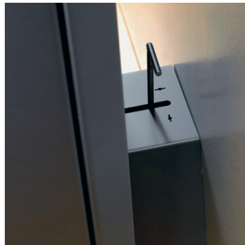
Shield and damper behind stove
